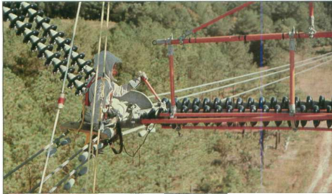
Fig. 2: A Linemen Wearing a Conductive Suit is About to Change a Insulator String
