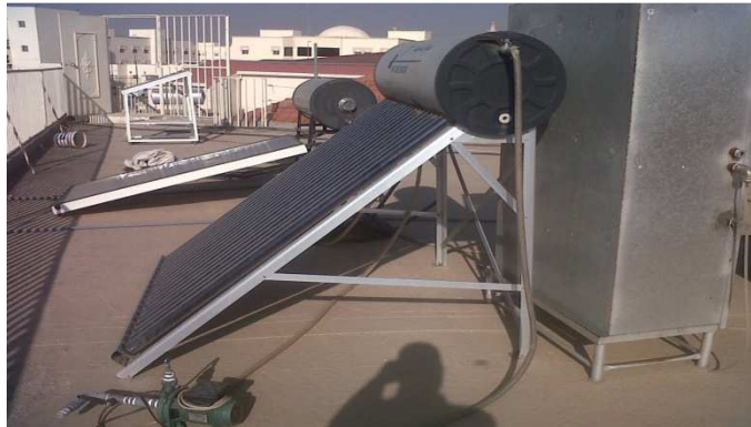
Figure 3: Photograph of the Solar Heating System
